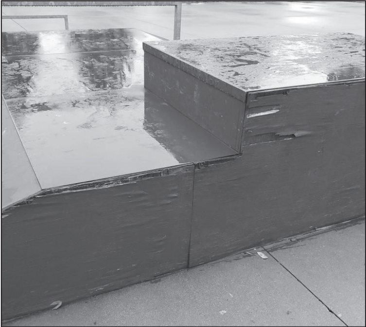
With repeated use, the wooden structures at the Lowell Skatepark have begun to break down. These features, now dilapidated, were originally part of a small grassroots effort to give Lowell a skatepark, but they were never meant to last forever.
