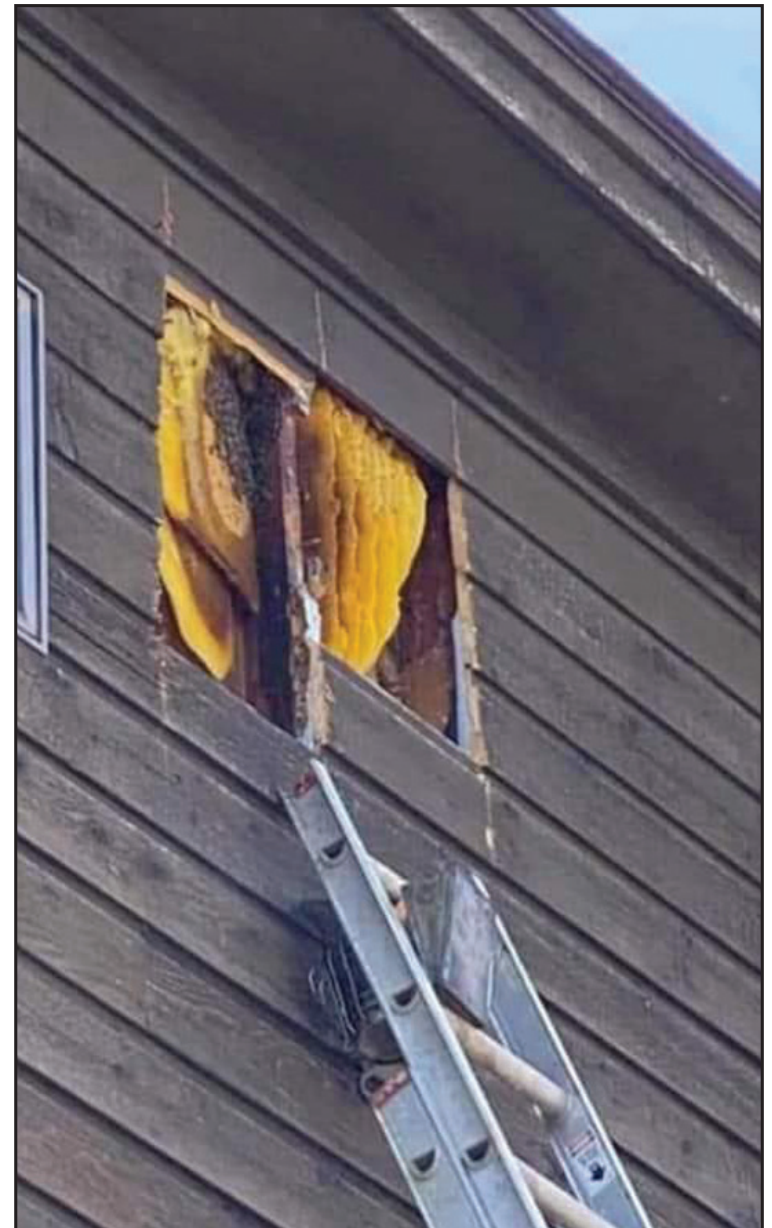
Cutouts in the walls. Photo Courtesy of Brown's Bee Service Facebook page.
