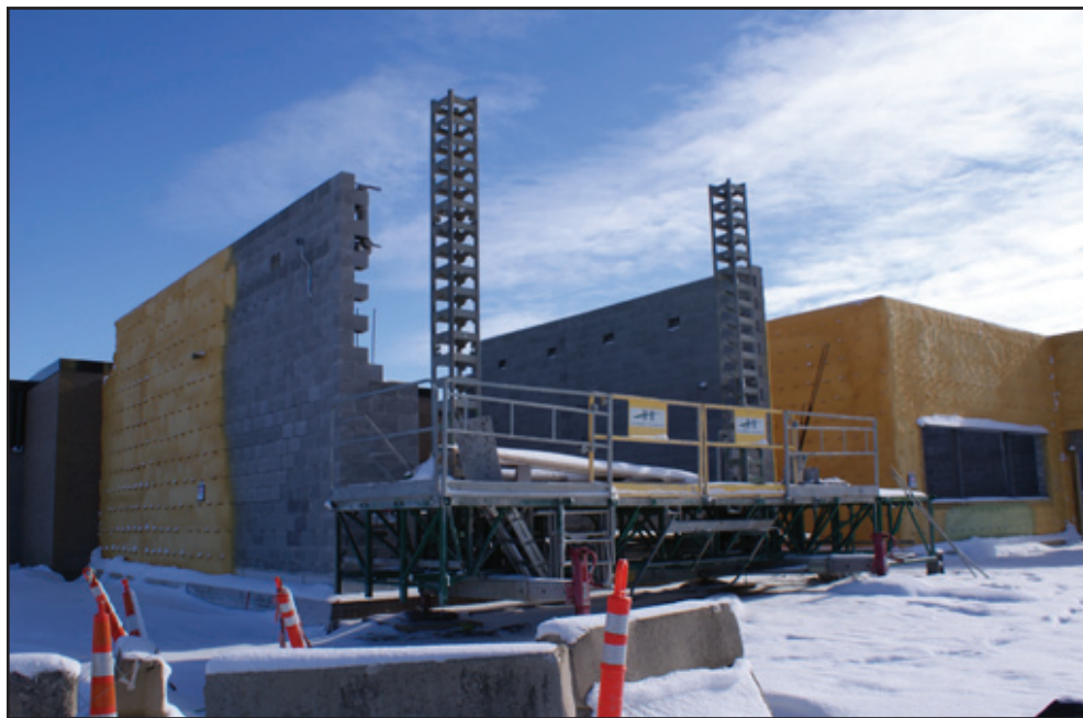
Exterior views of the new two story addition to Lowell Middle School.
