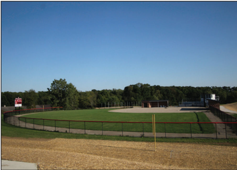
While the softball and baseball fields at LHS did exist prior to the construction, major improvements are being made including dugouts, scoreboards, and stands.
