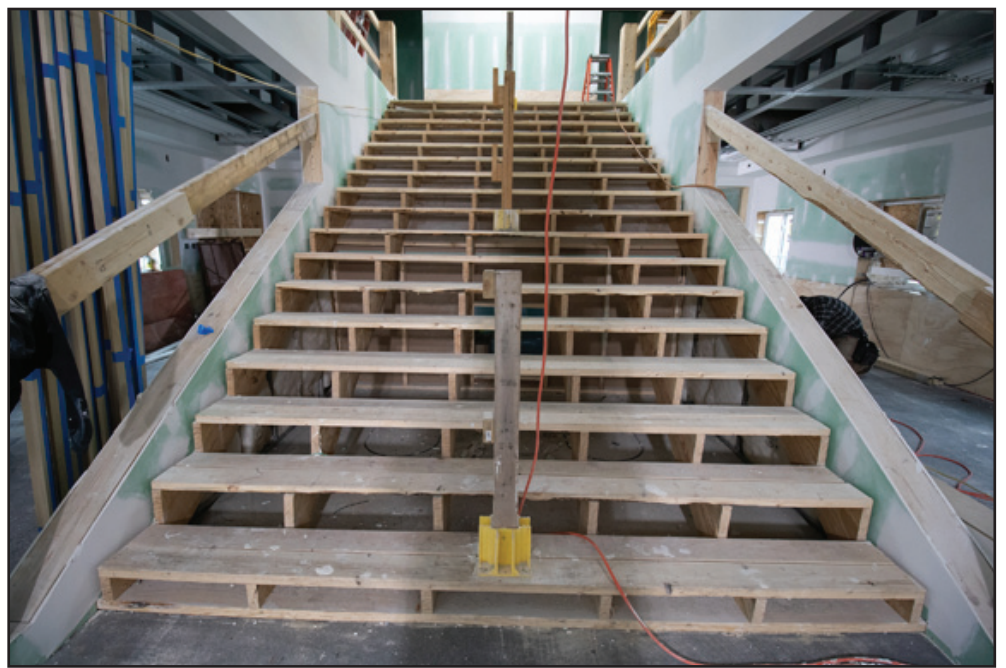
The custom staircase connecting the first and second floors still needs to be trimmed out. This will be the final task when Wolverine completes the interior of the Showboat.
