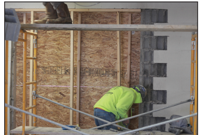
“The future main electrical room is being prepped for future installation of electrical equipment. Masons are infilling openings and tooting in masonry at future openings.”
