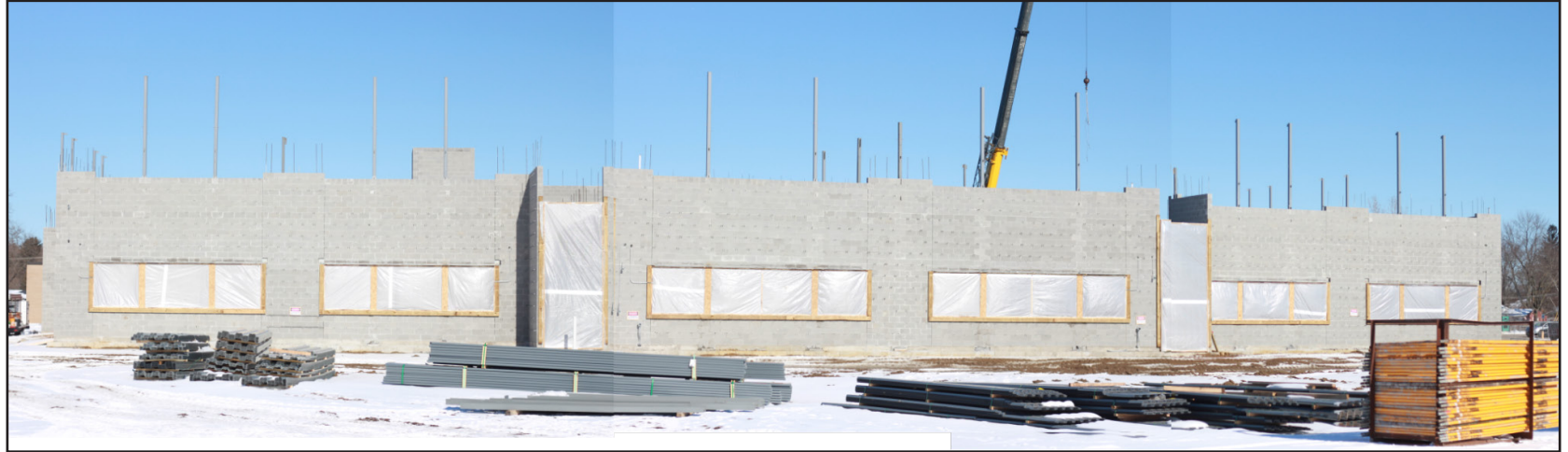
“Temporary window and door coverings have been built and installed to allow containment of heat for future slab pours. South face of the Unit D addition is pictured.”
