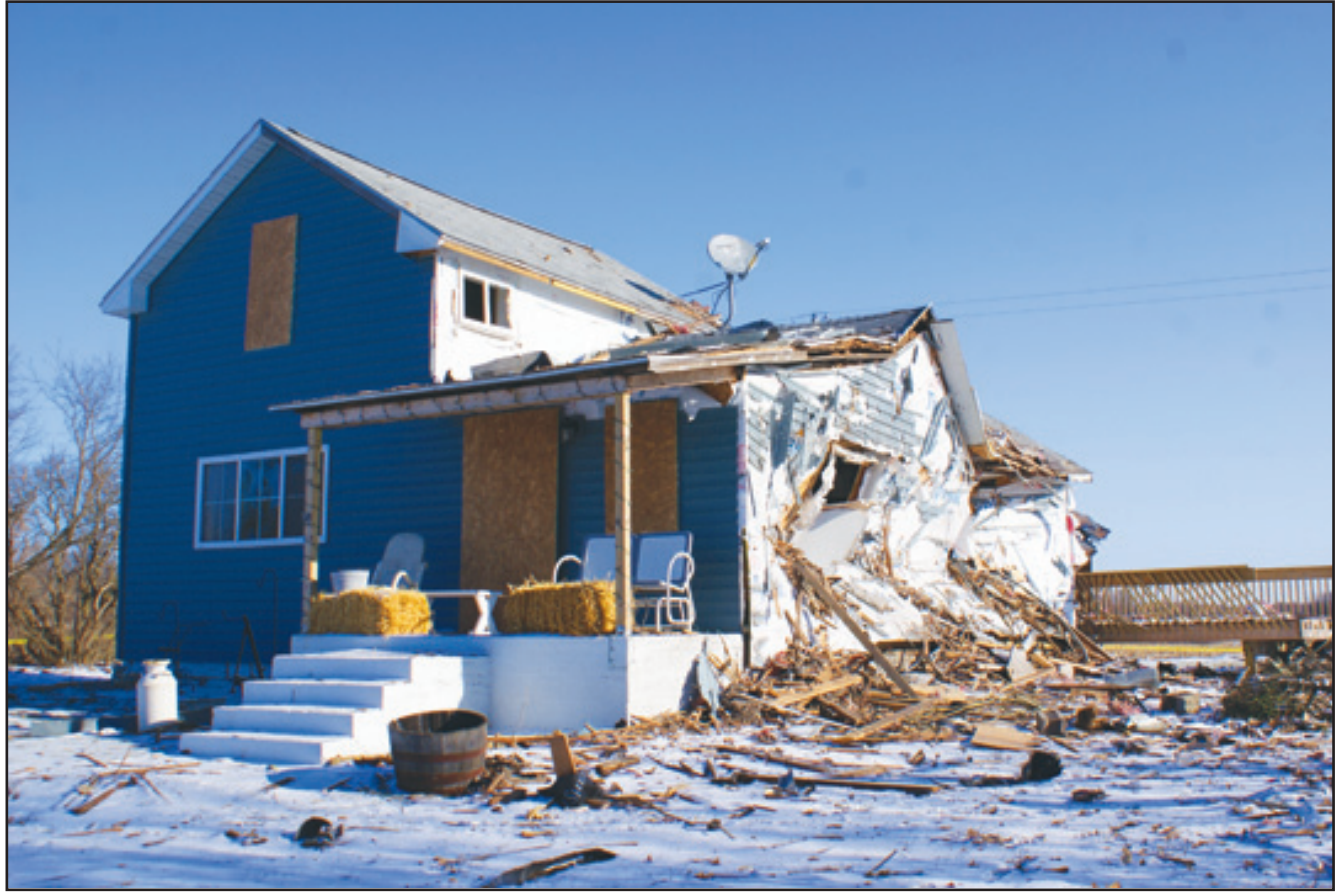
This house on Fallasburg Park Dr. exploded in the middle of the night on Monday, Dec. 16. The cause is under investigation.
