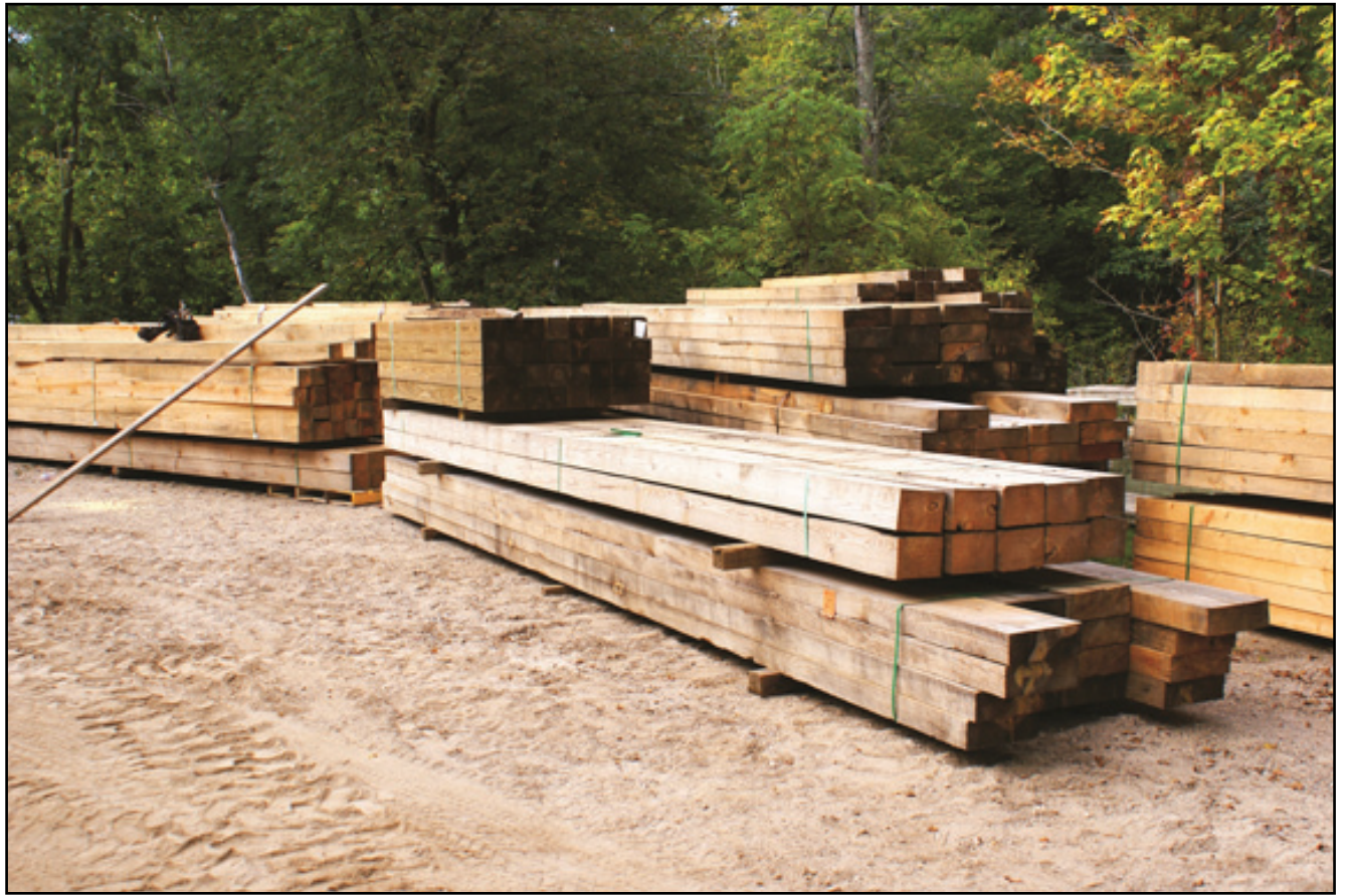
This pile of timber will be used to build a replica of Whites Bridge. The project is scheduled for completion in late December.
