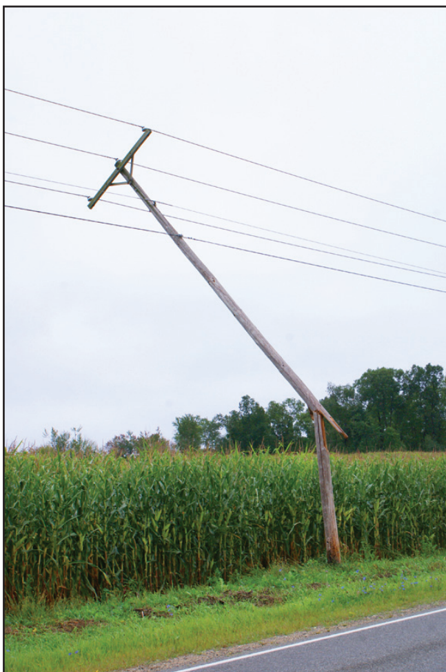
Wooden power poles like this one on Bailey Dr. were no match for the 100 mph winds. Many local residents lost power during the frightening storm.
