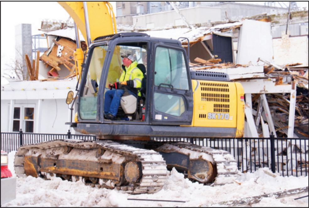
Earthworm Dozing and Excavating owner Dave Gonyon did much of the heavy work himself.
