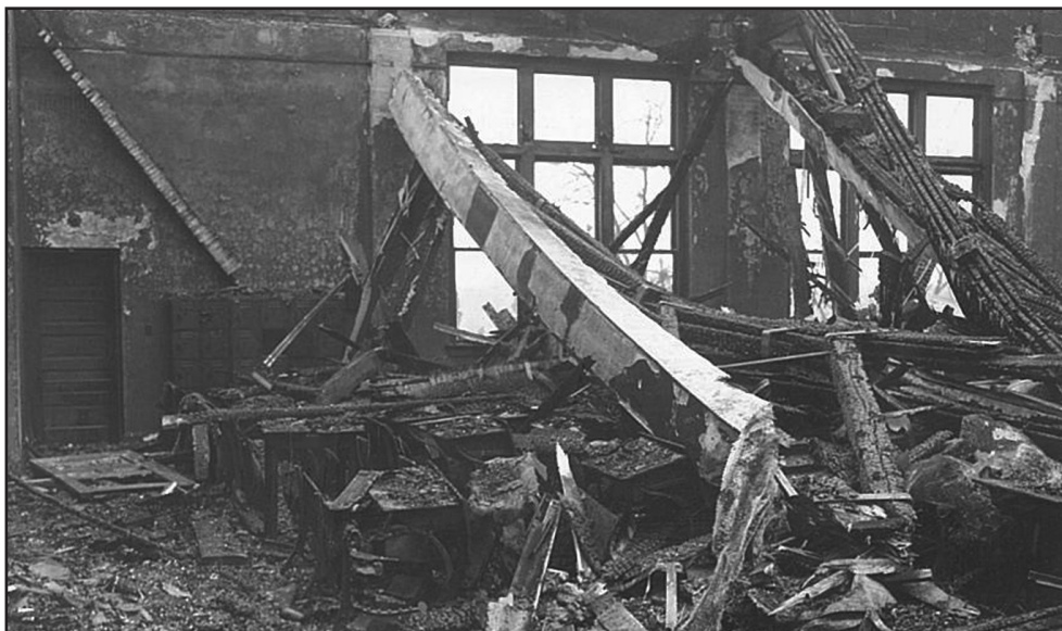
Lowell Ledger, Jan. 25, 1945: "The destruction inside the 30-year-old building can best be understood by this picture showing the roof as it collapsed on the rear of the high school session room." Photo by Leonard Studios, Lowell, courtesy of Flora Jean Beachum.
