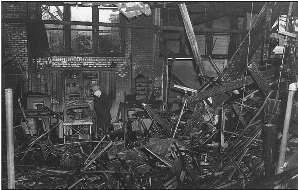
A fire inspector surveys the damage to a sixth grade classroom. Photo by Leonard Studios, Lowell, courtesy of Flora Jean Beachum.
