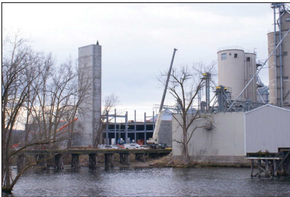
Above, construction of new facilities at King Milling is underway. Above right, a view of the work at the future Main St. location of Impact Church.
