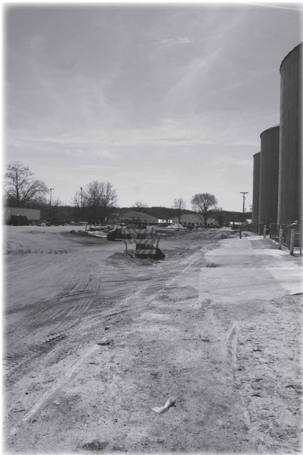
Construction on S. Broadway, near King Milling and the fairgrounds, should be finished in a couple months.
