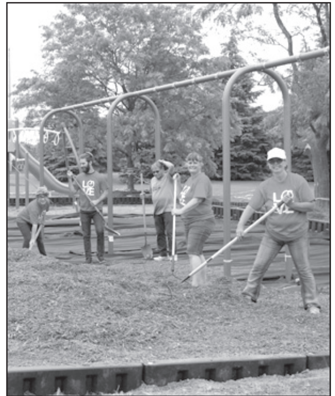
Volunteers were tasked with knocking down the old equipment and then digging out 12 inches of soil for new mulch.
