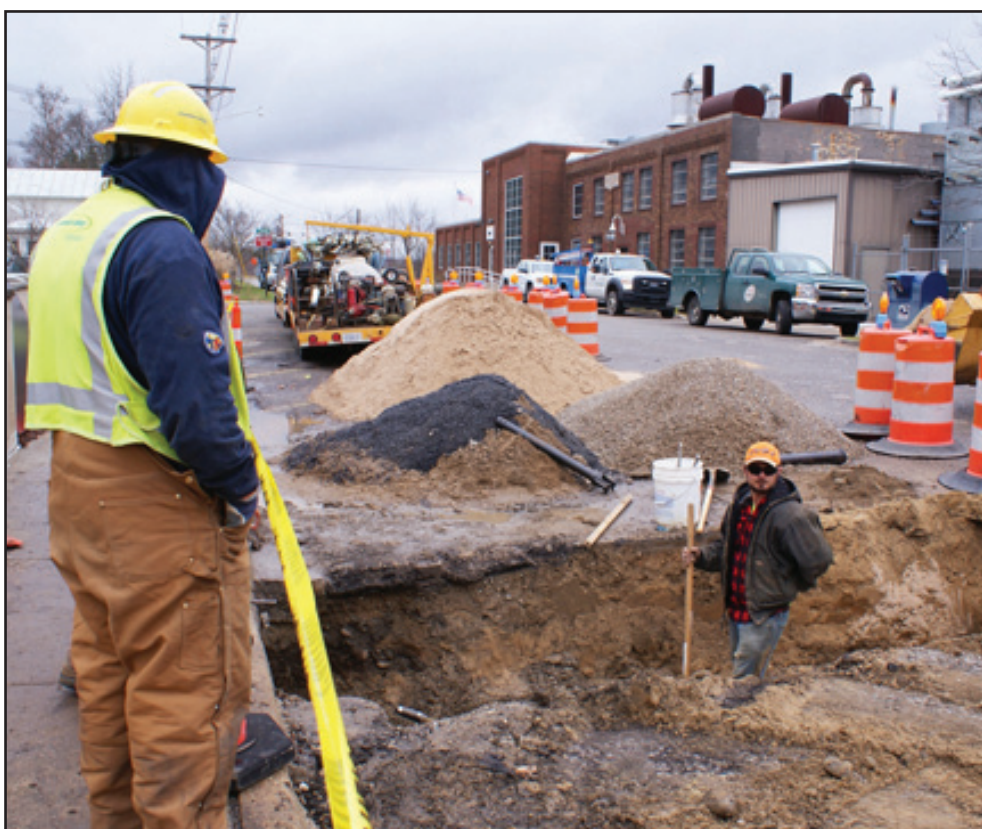
A crew from Consumers Energy fixing a gas leak on Broadway last Thursday.
