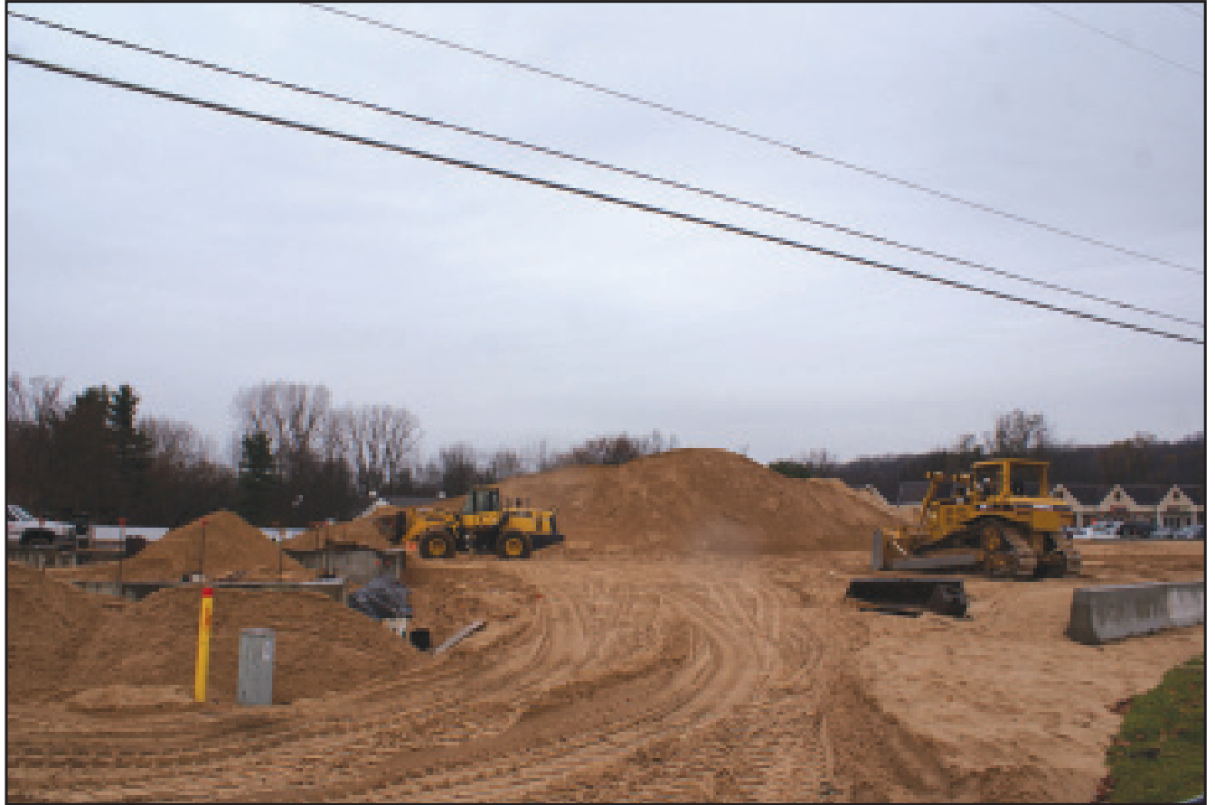
Construction on phase one of the Ada Village plan, a realignment of Headley St., started in July and is due to finish in December.
