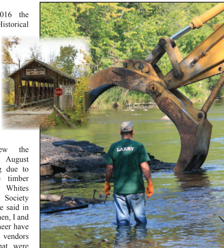
Inset: A stock photo of Whites Bridge before the fire and above, crews removing remnants from the Flat River in August 2013. (Ledger Aug. 20, 2013)
