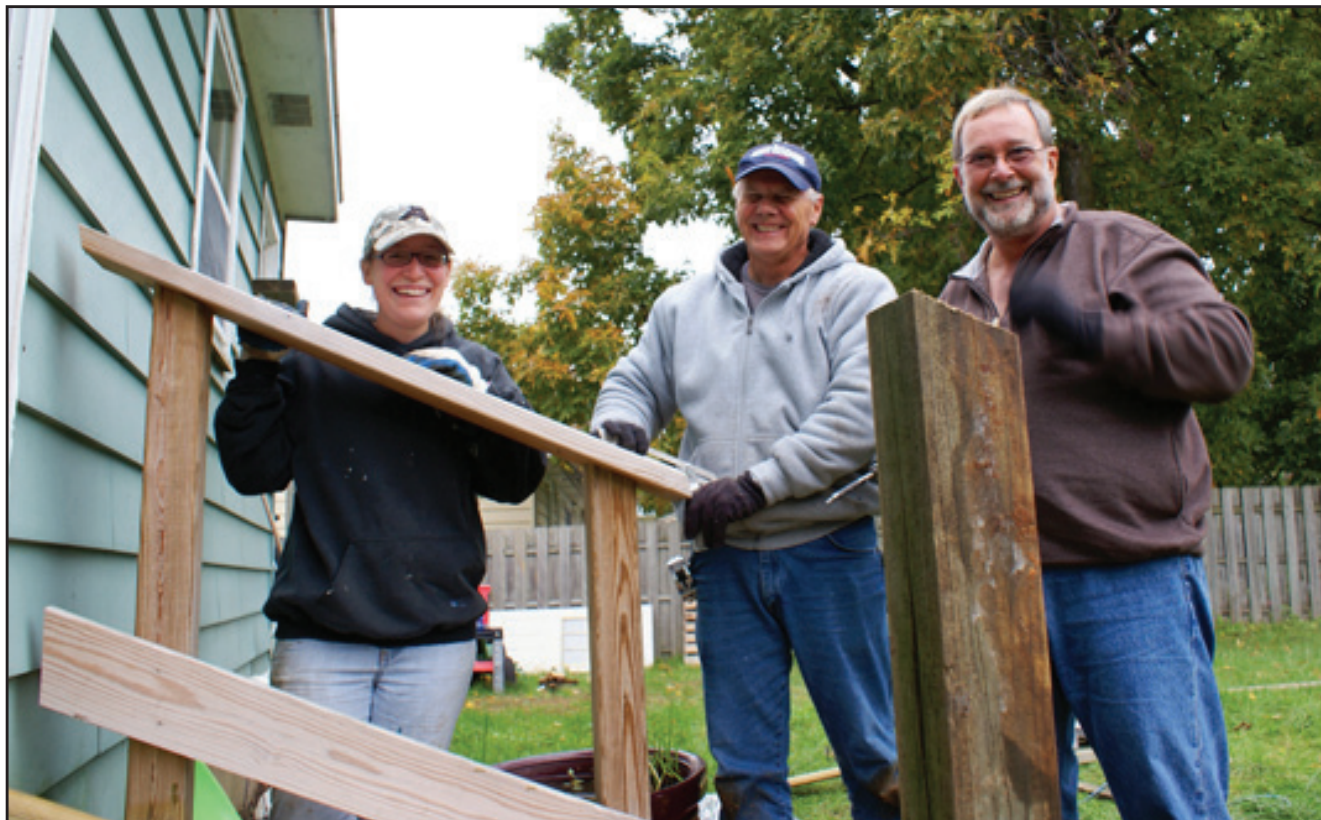
Karen Noreen, John Sterly and Jim Hodges built new stairs on the back of a house.
