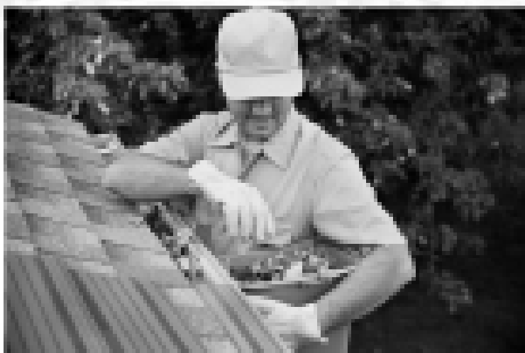
• Single mother needs gutter cleaned. She is physically unable to climb a ladder.
