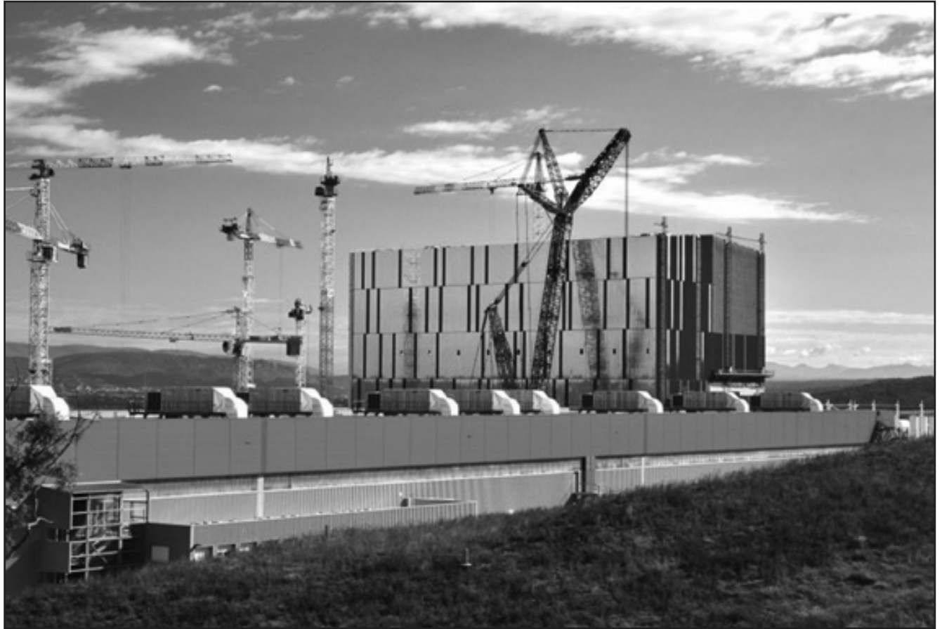
The EU, US, China, India, Korea, Russia and Japan have all contributed to the ITER fusion reactor currently under construction in southern France.
