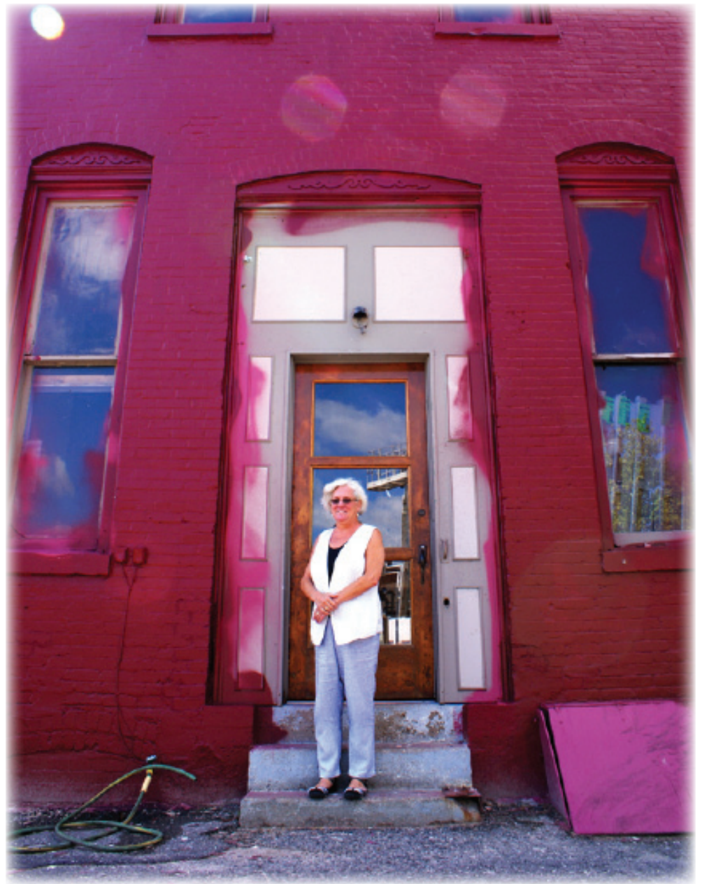
LowellArts! executive director Lorain Smalligan is asking for the public’s help to finish remodeling their new Main St. location.
