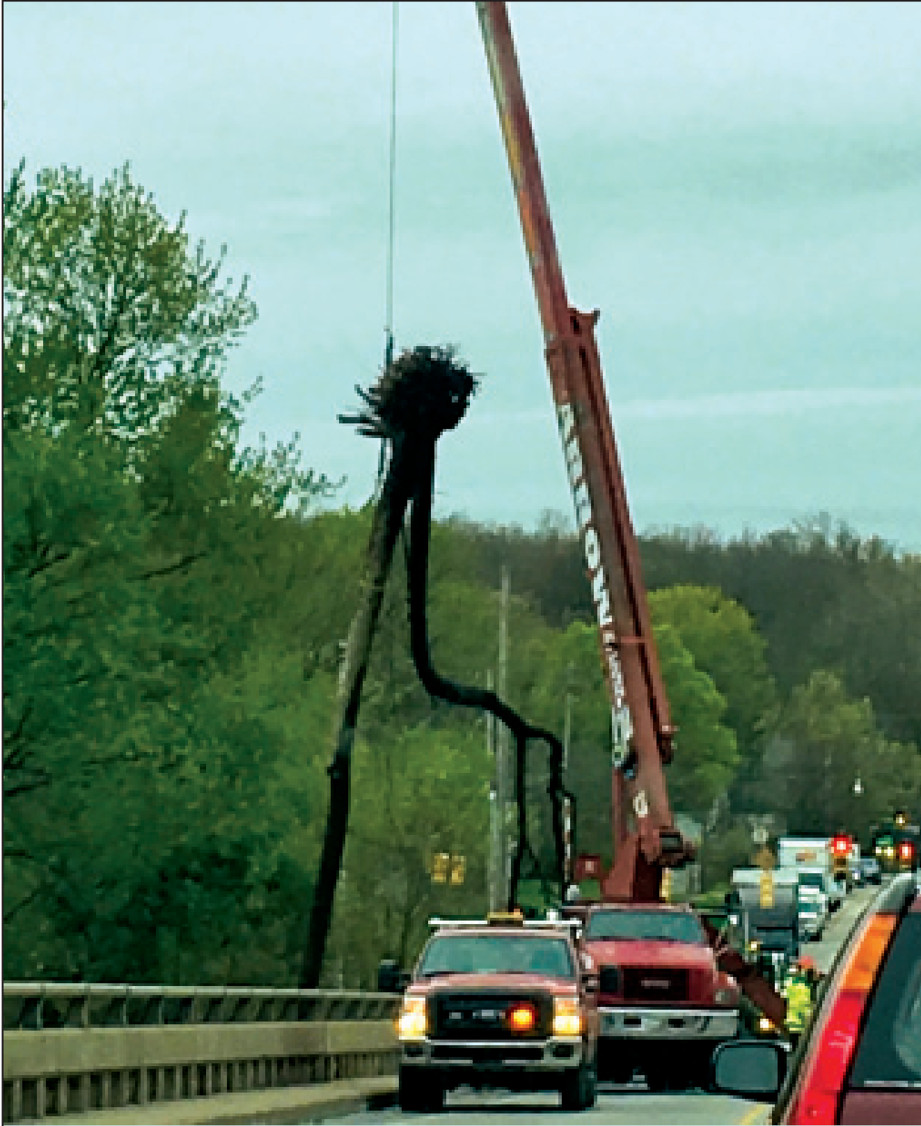
Lisa Davis submitted this picture of Tuesday morning's stalled traffic. The backup caused by a crane on the bridge removing a tree from the river. Vehicles were stopped north of Main Street on Alden Nash all the way to Grand River.
