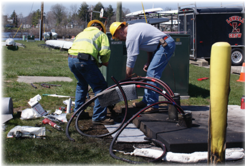
Lowell Light & Power employees worked to restore power as soon as possible.
