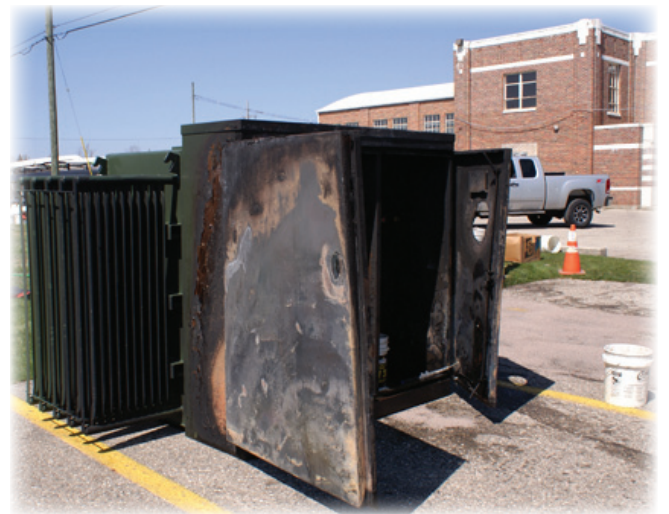
The burned out transformer a couple hours after the fire.
