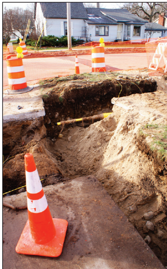
Gas lines were replaced by Consumers Energy on Bowes Rd. last week.
