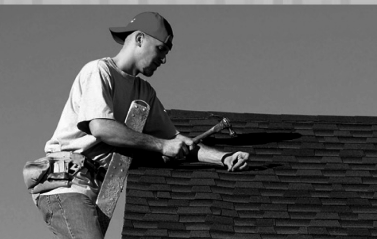
• Senior citizen's roof leaking over the bedroom and bathroom. Some damage inside home too.
