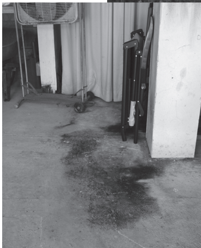
Scorch marks on the floor show there was a fire in the garage.
