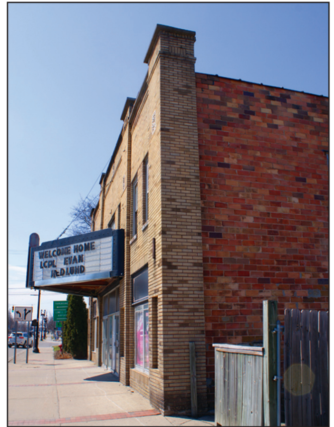
The marquee from the historic Strand Theater is still in place. The exterior walls had to be pulled together after a truss fell down.
