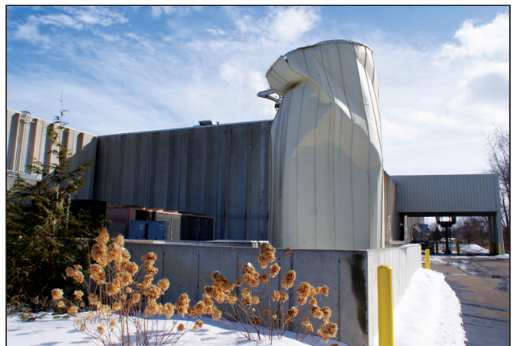
The damaged silo outside at Litehouse Foods.
