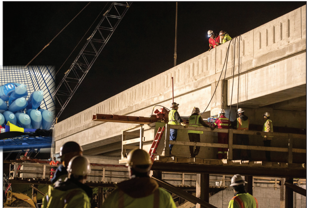
The bridge slide project was completed with the help of Dawn dish detergent.
