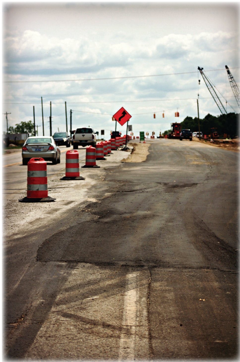
Traffic continues to flow freely over the existing M50 bridge while finishing touches are being put on the new one.
