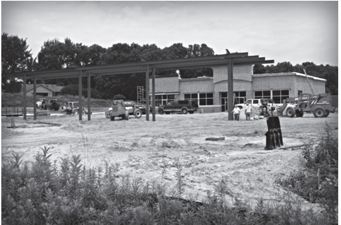
Construction crews continue to work on the new gas station and restaurant slated for an August 28 opening.
