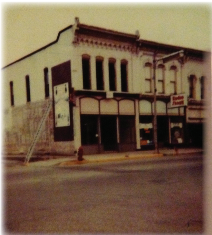
The building in the process of renovation and, at right, newer storefronts.
