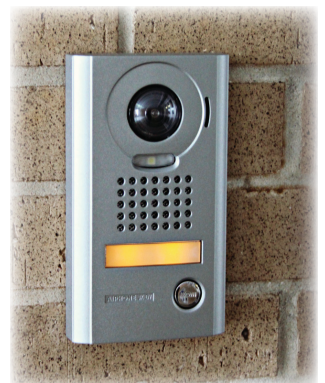
Audio and video equipped buzzer entry systems have been installed in elementary buildings.
