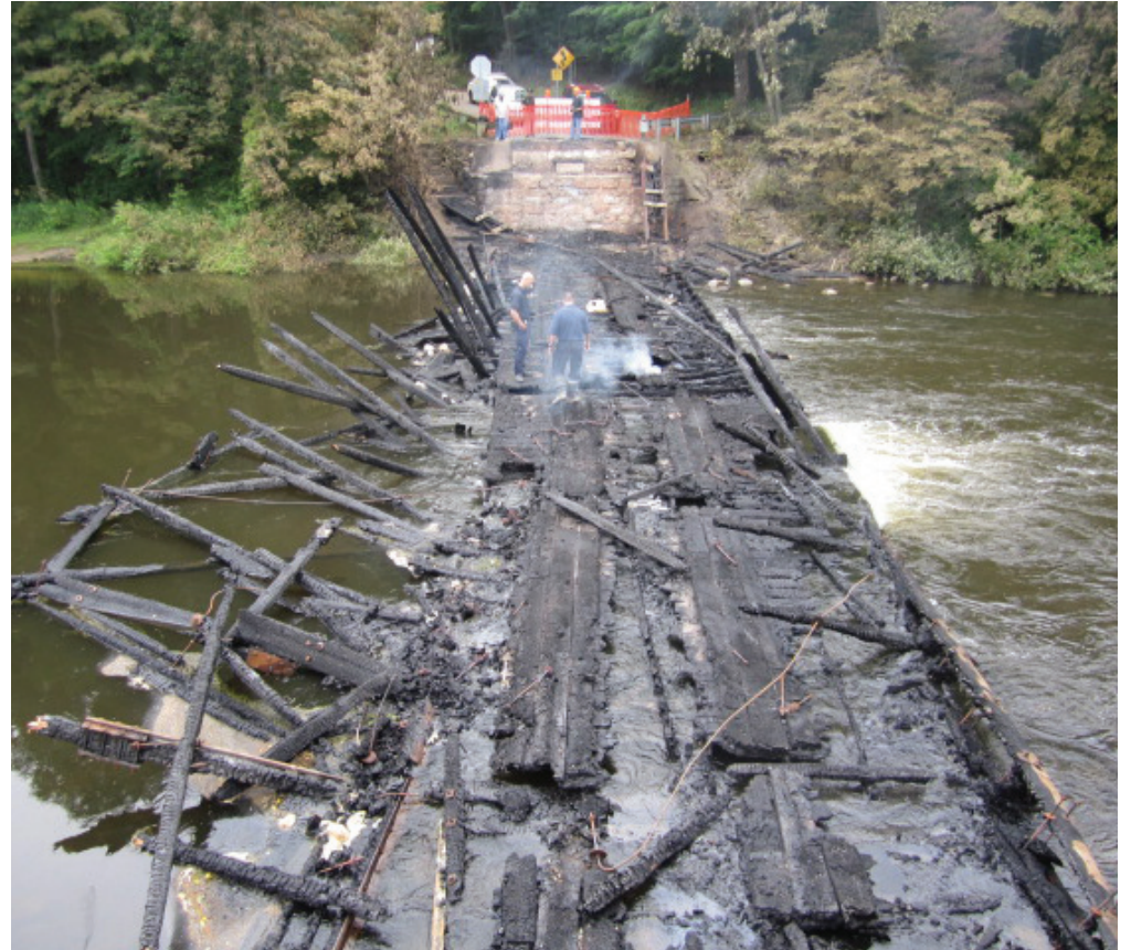
Only the stone abutments on either end of the bridge can be salvaged for a new bridge, Ionia Road Commission says.
