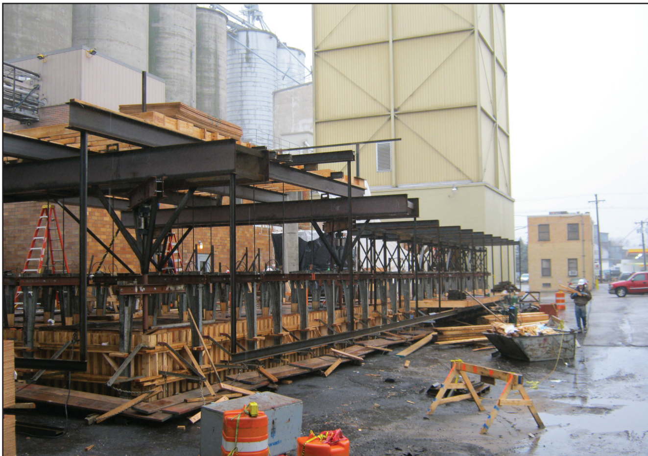
The beginning stages of the building process, before the concrete walls have been poured.
