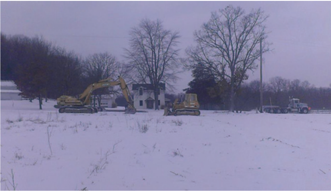
Construction began a month ago on the new drive thru feed store
