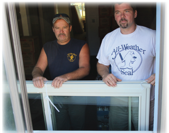
Al Norton and Tony Perkins of All Weather Seal install the 26 windows in the courtyard of Flat River Outreach Ministries.
