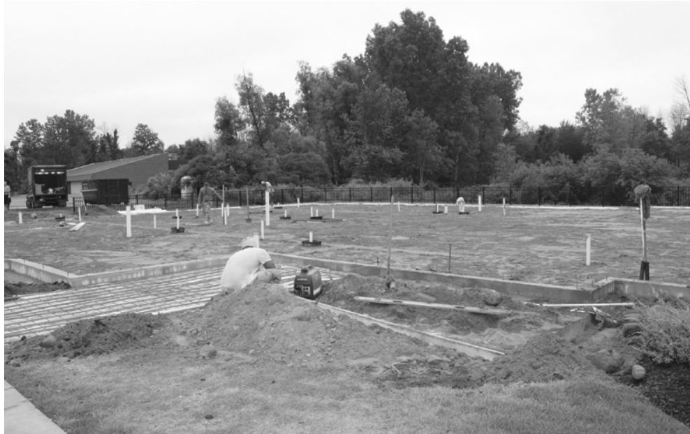
The memory care addition to Green Acres is slated for November completion.
