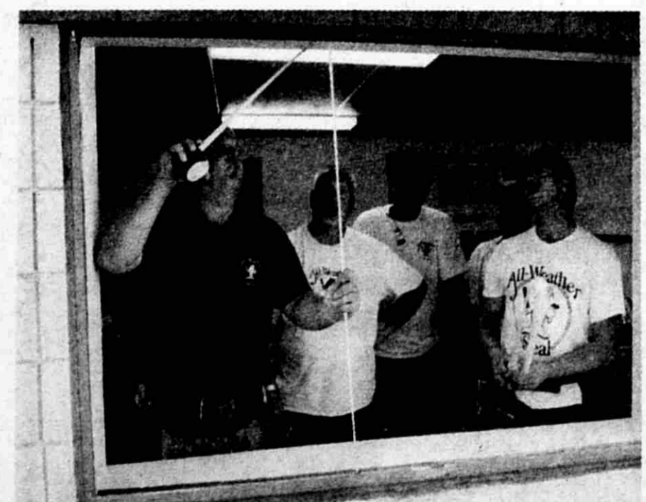
All-Weather Seal crew, George Banfill, Mickey Thompson, Tony Perkins, Al Norton and Eric Bergmans, installed windows at FROM.
