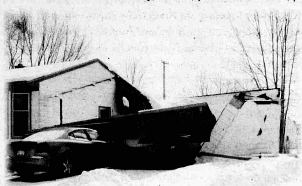
This roof over a garage at a rental home on Valley Vista Drive collapsed due to heavy snow.
