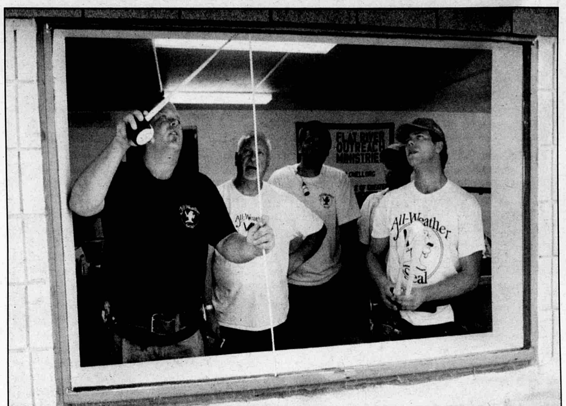
All-Weather Seal crew, George Banfill, Mickey Thompson, Tony Perkins, Al Norton and Eric Bergmans, installed windows at FROM.
