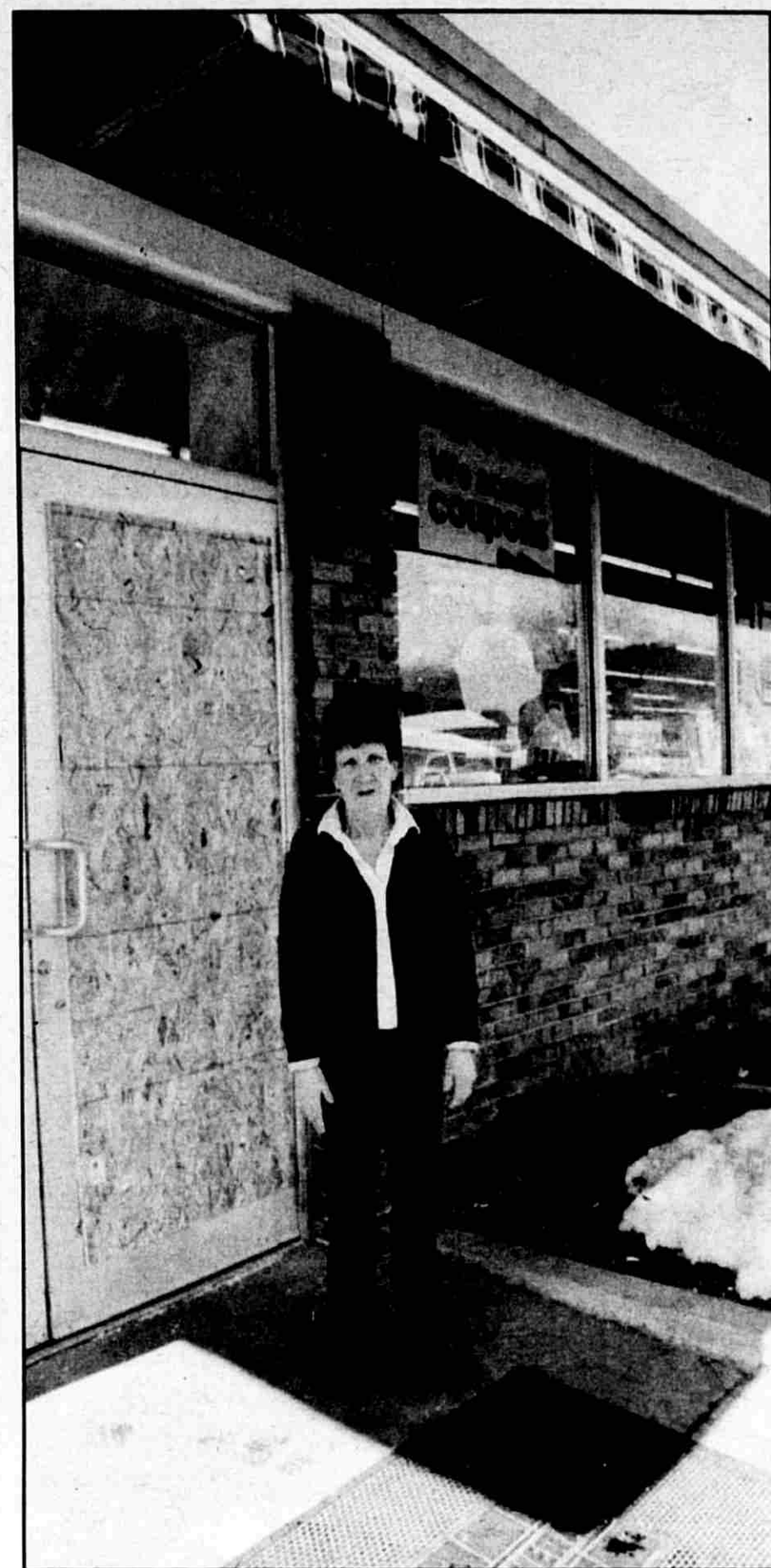
Manager Anna Smith stands by a boarded up door panel at the Dollar General store on Monday.
