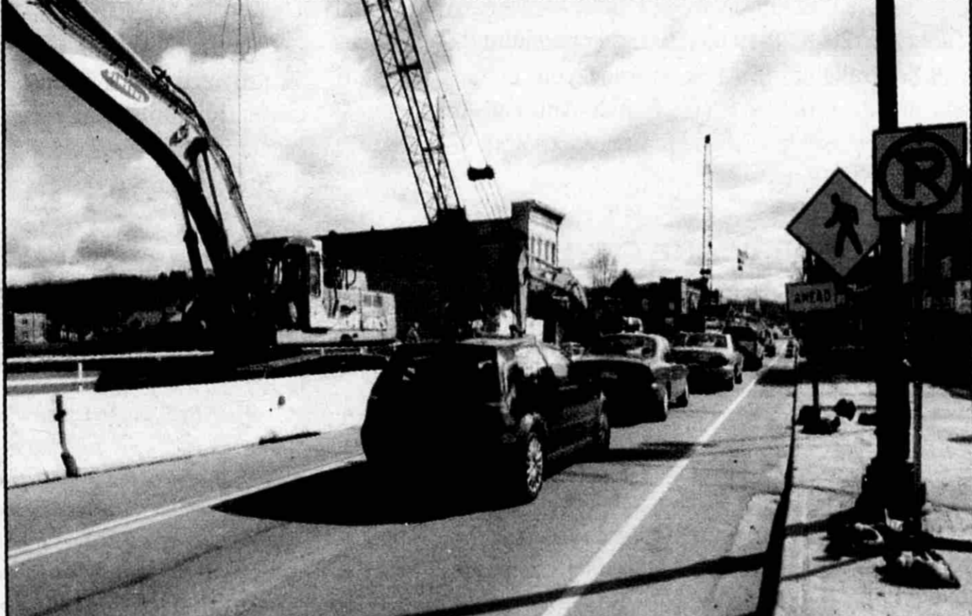
A concrete barrier wall separates the work zone from the eastbound traffic on the bridge.
