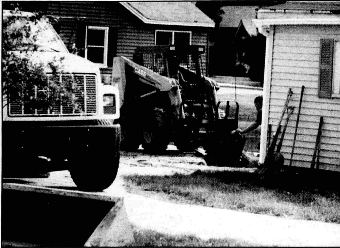
Local excavator, Stormzand Asphalt, helped state officials by removing the concrete patio.
