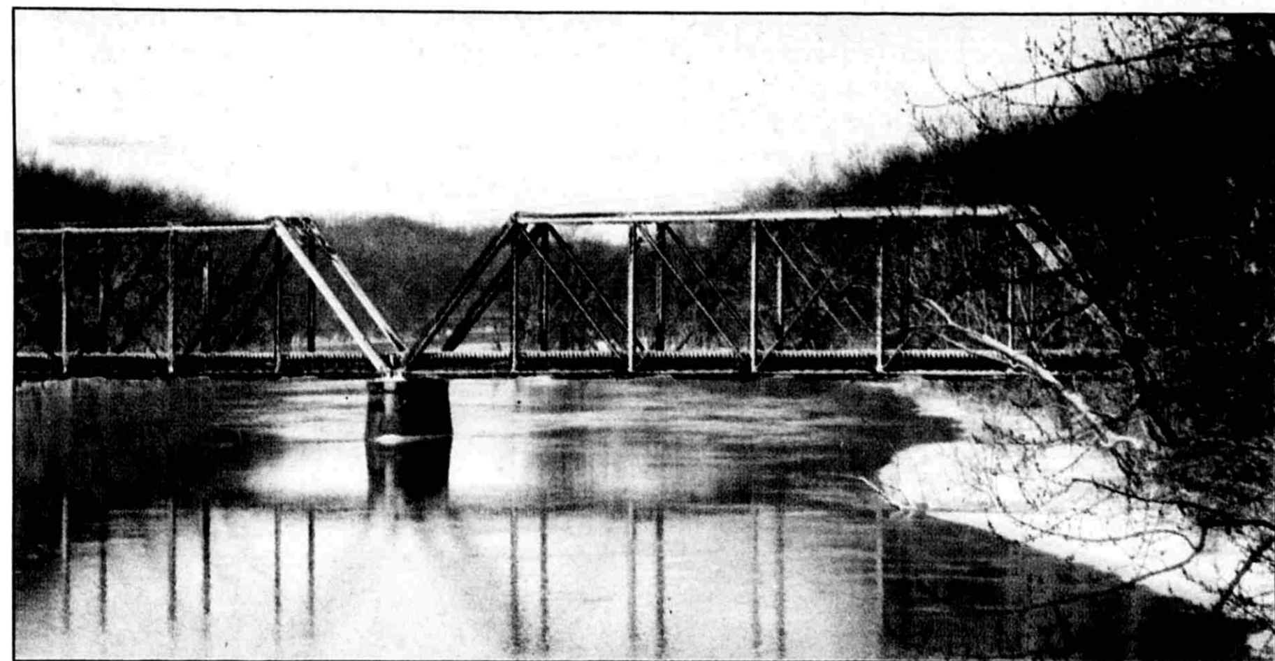
This railroad bridge over the Grand River is one of many structures on the railroad corridor.
