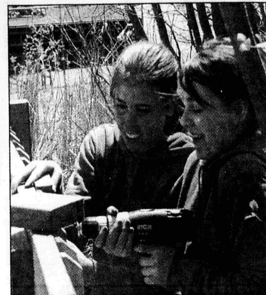
Lowell High School freshmen Tricia VanGessel, left, and Lauren Wolfe assemble a railing for a wheelchair ramp at Camp Tuhsmehta, a summer camp for the blind in Greenville. 5-3-06
