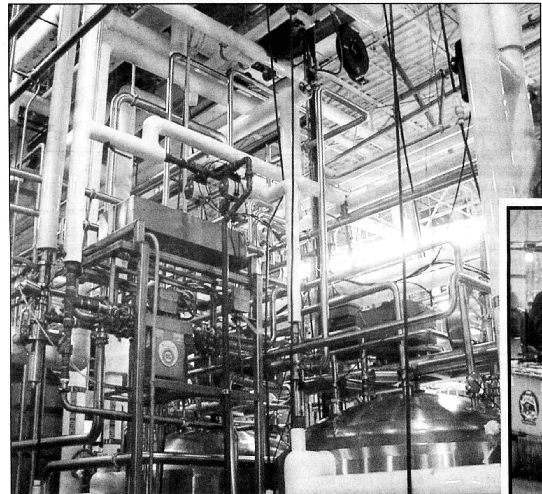
A complex network of pipes carries canola oil, buttermilk and other bulk ingredients to the mixing station on the production floor.
