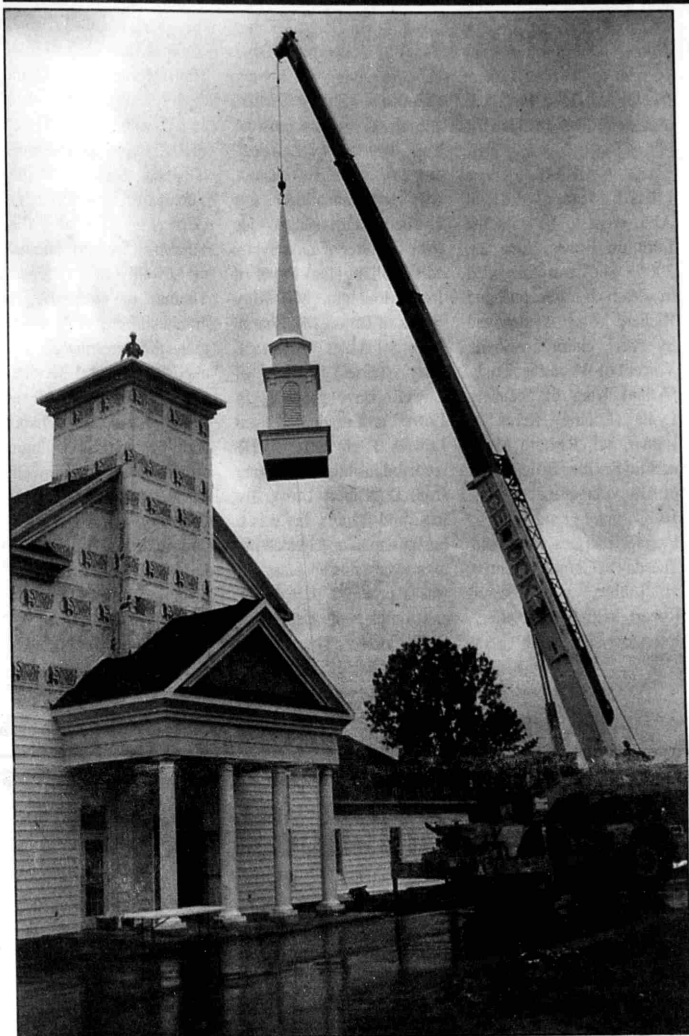
A crane lifts the steeple to the top of the First Congregational Church of Lowell's new sanctuary on Lincoln Lake Ave.
