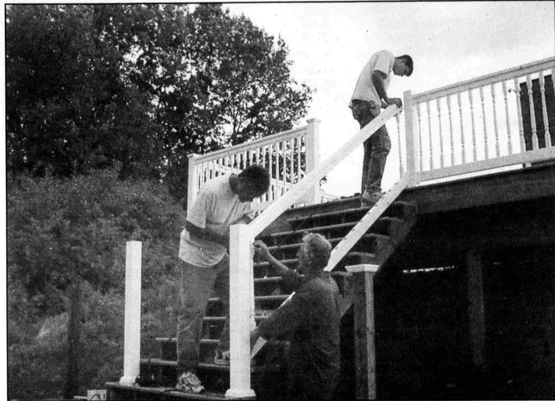
Bill VanderKlok, left, Jack VanderKlok, right, and Andy VanderKlok, top, install a railing on the observation deck, part of a memorial at Lowell High School for classmates who have passed away before their time.
