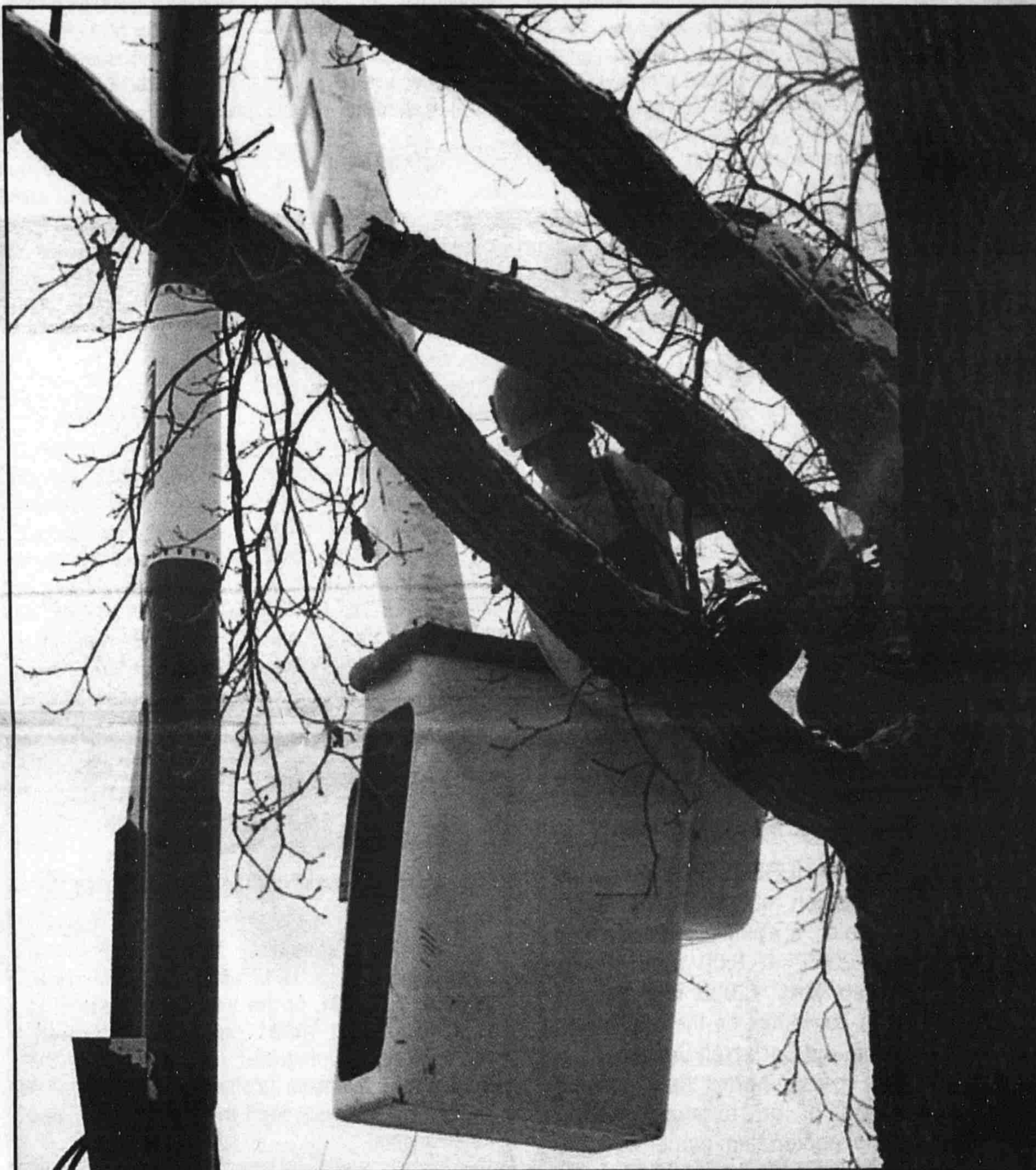
A worker with the Medco tree cutting company saws a limb from an oak tree on Bowes Road. Several trees are being felled on Bowes Road to make way for new power lines.
