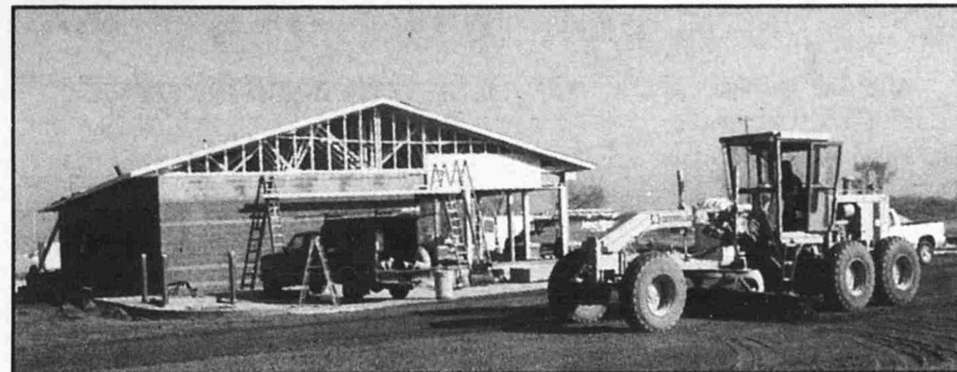
Construction has been underway for some time on a Mobil station on Alden Nash south of Cascade Road.
