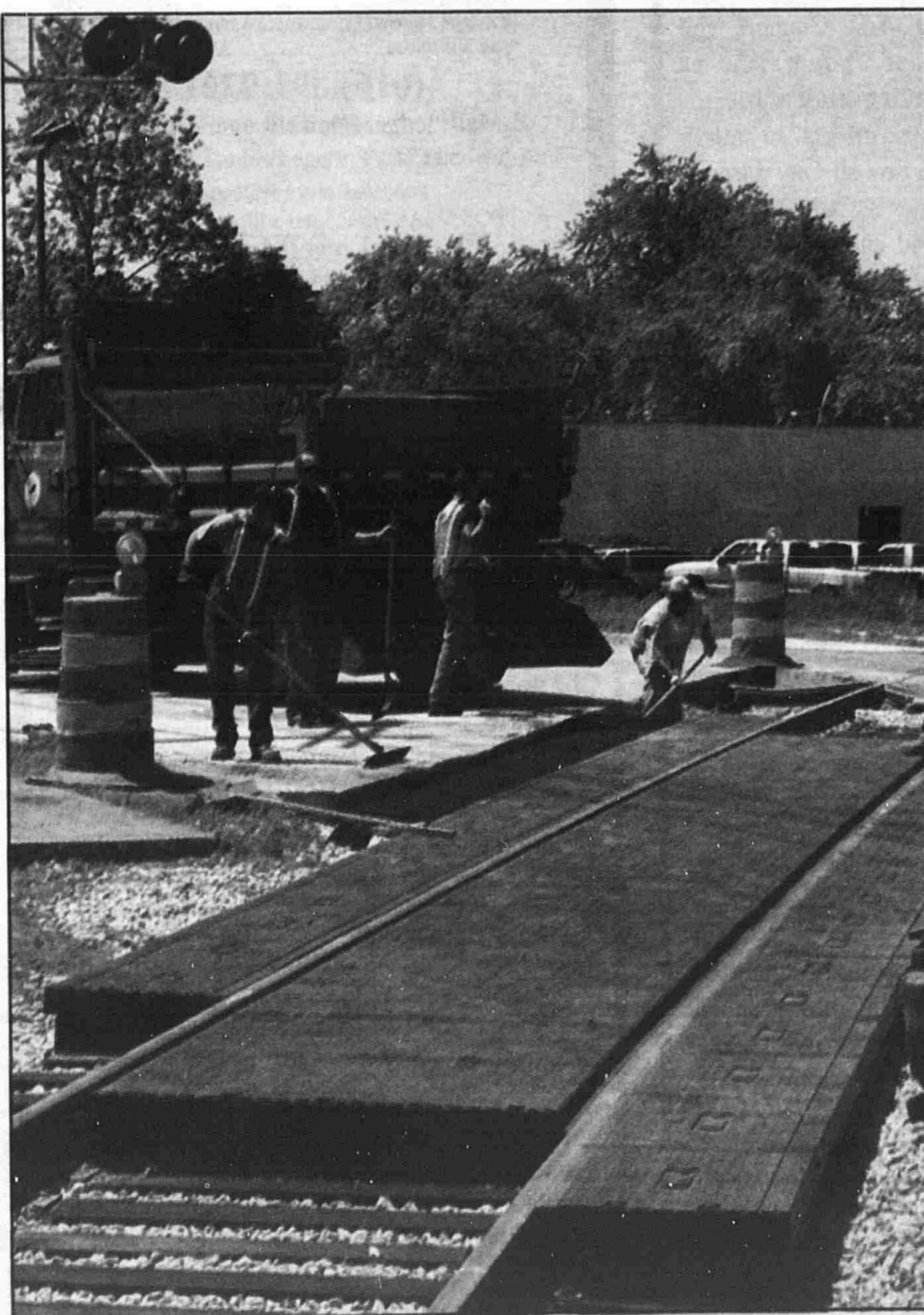
A Kent County Road Commission crew installed asphalt last week at the rebuilt railroad crossing on Main Street west of downtown.
