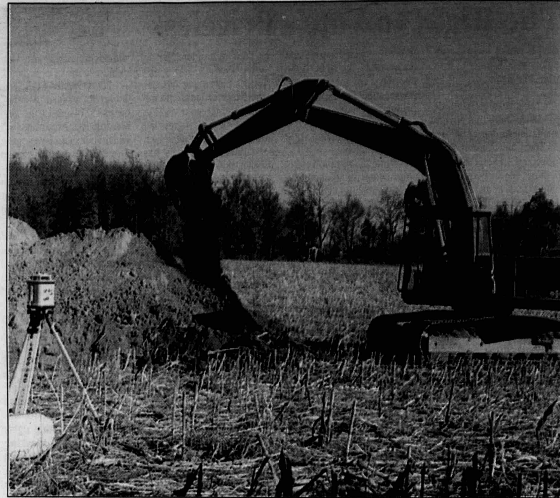
An excavator operator digs into the ground to allow the installation of drainage tile on farmland in southeastern Lowell Township. The excavation cuts through an area of Parkhill loam soil, which drains poorly compared to the Marlette loam soil that surrounds it.
