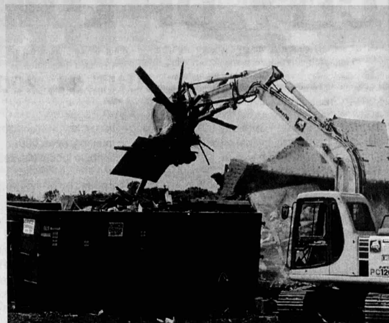
An excavator with a demolition claw pulls a load of debris from what was left of the Barton house last Tuesday.
